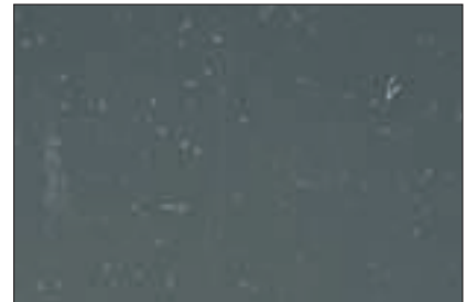
The joint has only been altered at isolated points by the UV-radiation.
