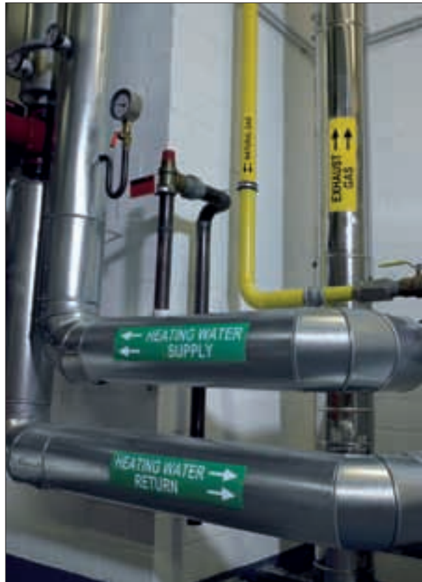
Large and highly visible pipe marking.
